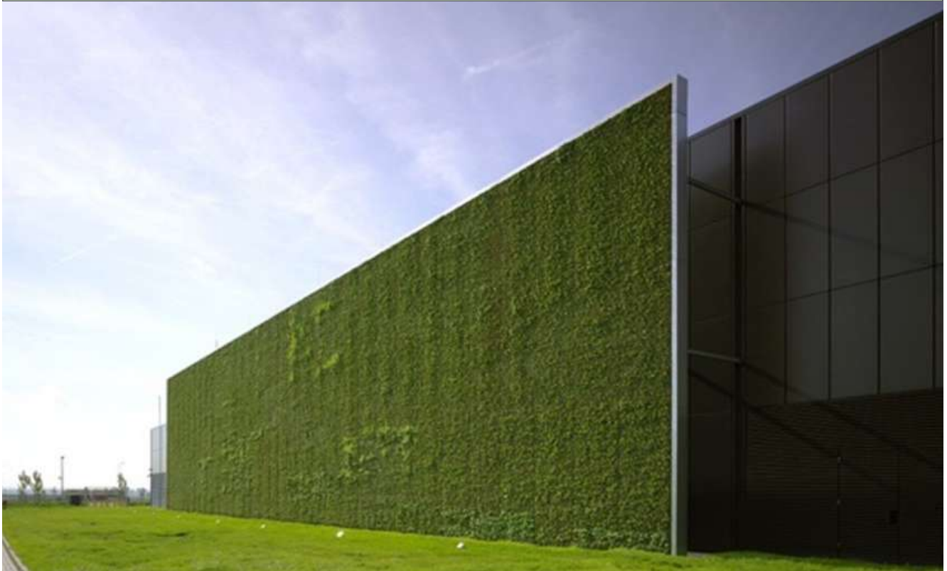
Figure 41: Green wall system (Frankfurt). Source: Arup, © Christian Richters
